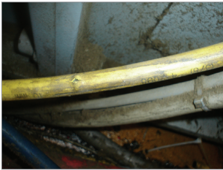
Multiple compressed air leaks can be found on holes present in shop tubing and fittings.
