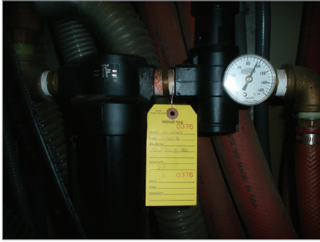
Air Leaks on FRL's
